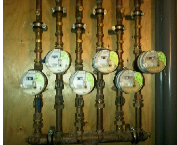
Manifold and Meters
